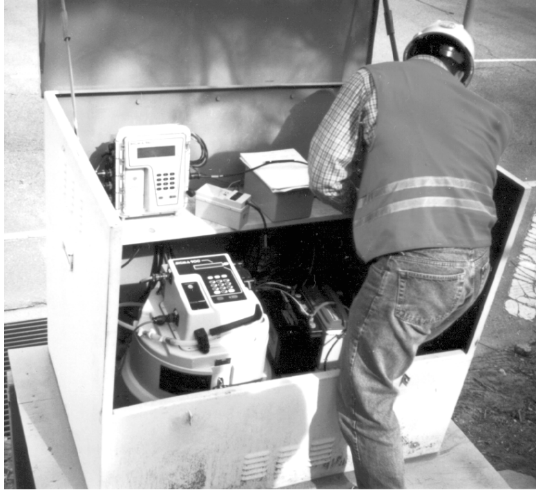
Figure 7-5. Automated Sampler Installation
