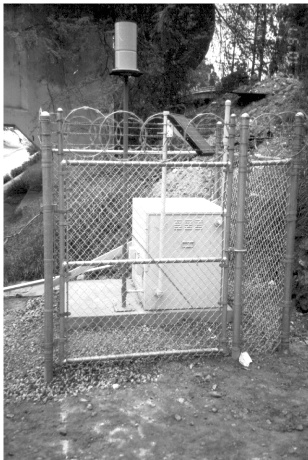
Figure 7-1. Example of Equipment Security
