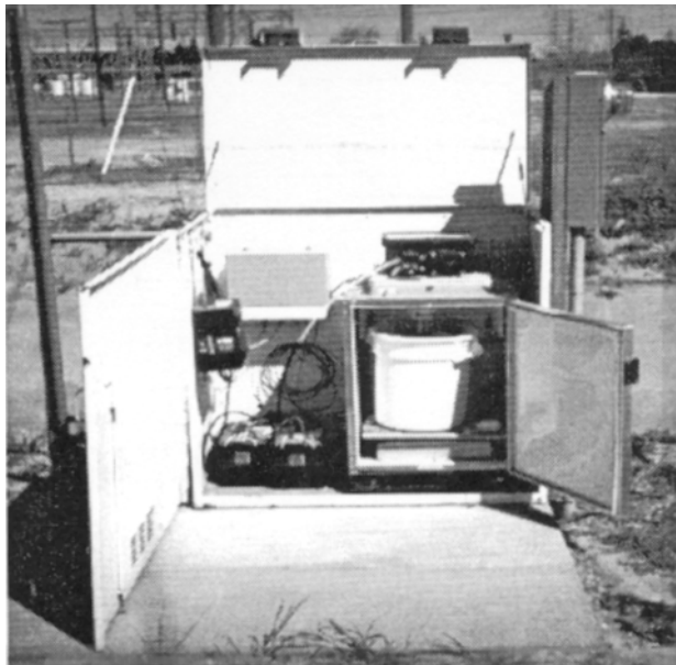
Figure 7-2. Steel Box Monitoring Station Enclosure
